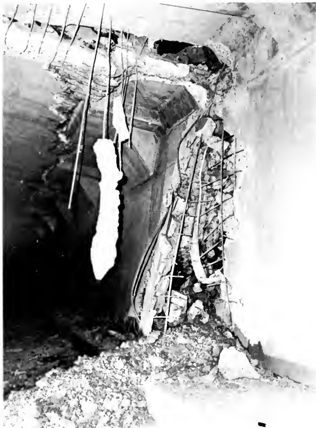
Photo 7. Joseph Jensen Filtration Plant, finished water reservoir. View of west wall, toward south. Metropolitan Water District photo.
